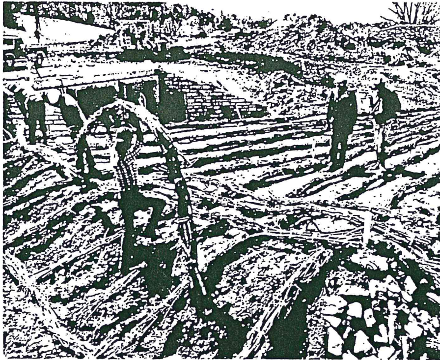
Workers on the Cumberland Gap Tunnel Project site place live fascines (bundles of living plant material) on the live boom, a soil bio-engineering project which is being constructed to redirect the stream of Little Yellow Creek. Alton Simms, (left, background), Vice President of the Soil Bio Engineering Corp., and Barry Carnes, field inspector with Vaughn & Melton, oversee the work.
